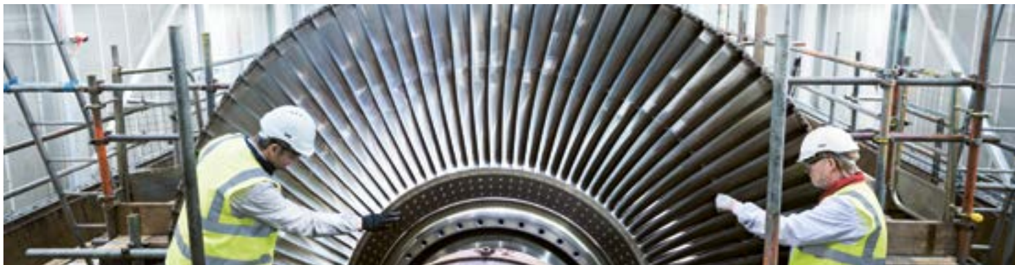
Engineers check the steam turbine in a gas-fired power station. Combined cycle gas turbine power stations use both a gas turbine and a steam turbine to generate electricity.
