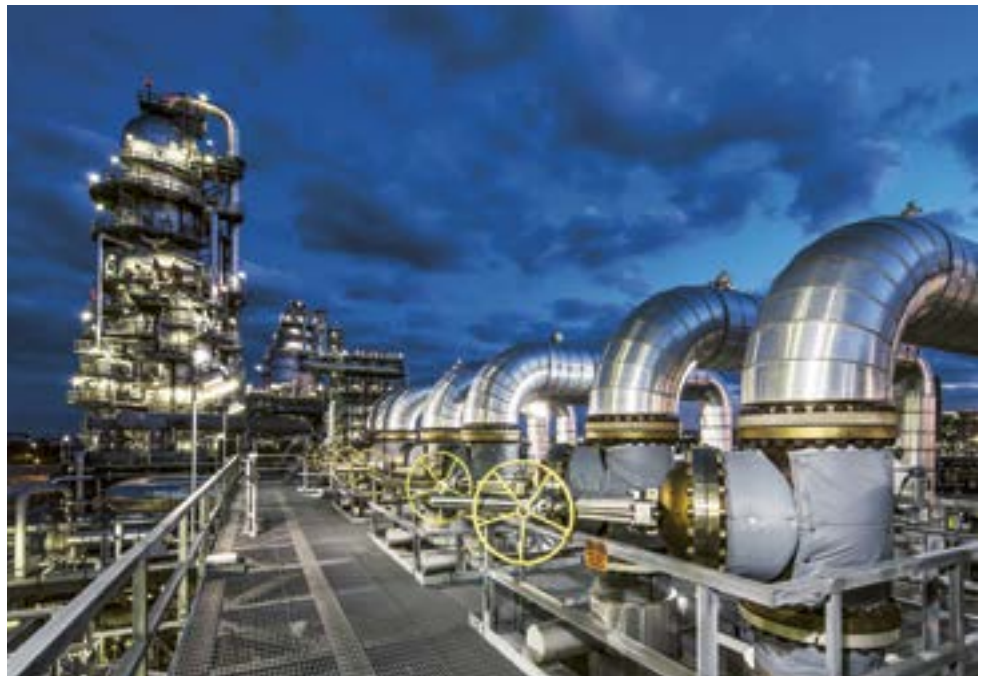
BP's Whiting Refinery – refineries are expected to benefit more from digitization and other advances that improve efficiency than from transformational changes in technology.
