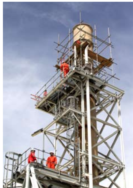
People at work at the BTC pump station 2 in Georgia
