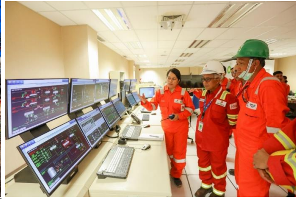
Main control building of Tangguh production
